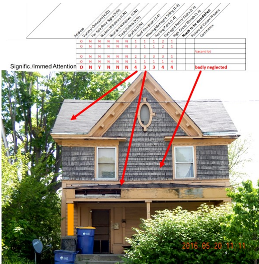
Figure 3B: Housing Sample, “Significant/Immediate Attention” category
